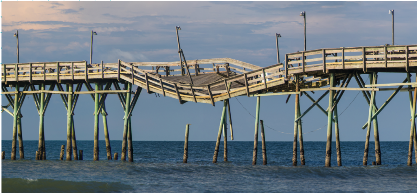
Pier damaged by Hurricane Isaias in Ocean Isle Beach, North Carolina.
