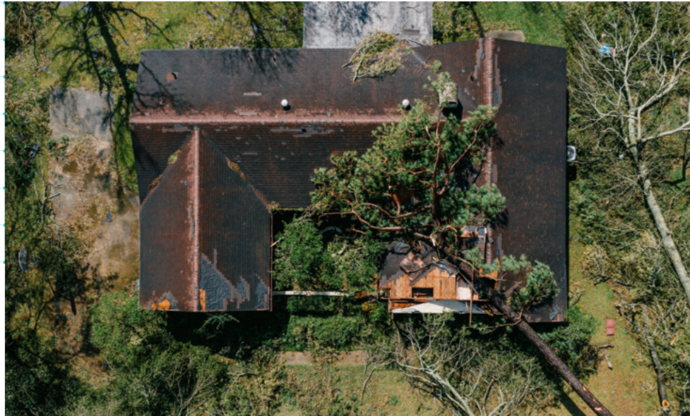
Aerial view of a house damaged by a fallen tree after Hurricane Laura made landfall in Lake Charles, Louisiana.
